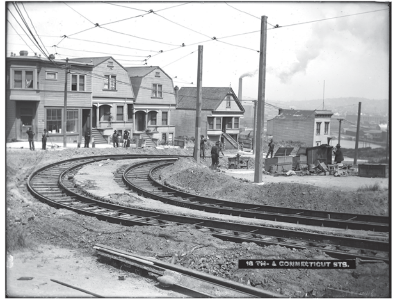
Streetcar tracks being installed at 18th and Connecticut streets on June 27, 1905. Today, Sunflower Vietnamese Restaurant occupies the building to the far left. PHOTO: Courtesy of SFMTA.com/Photos
