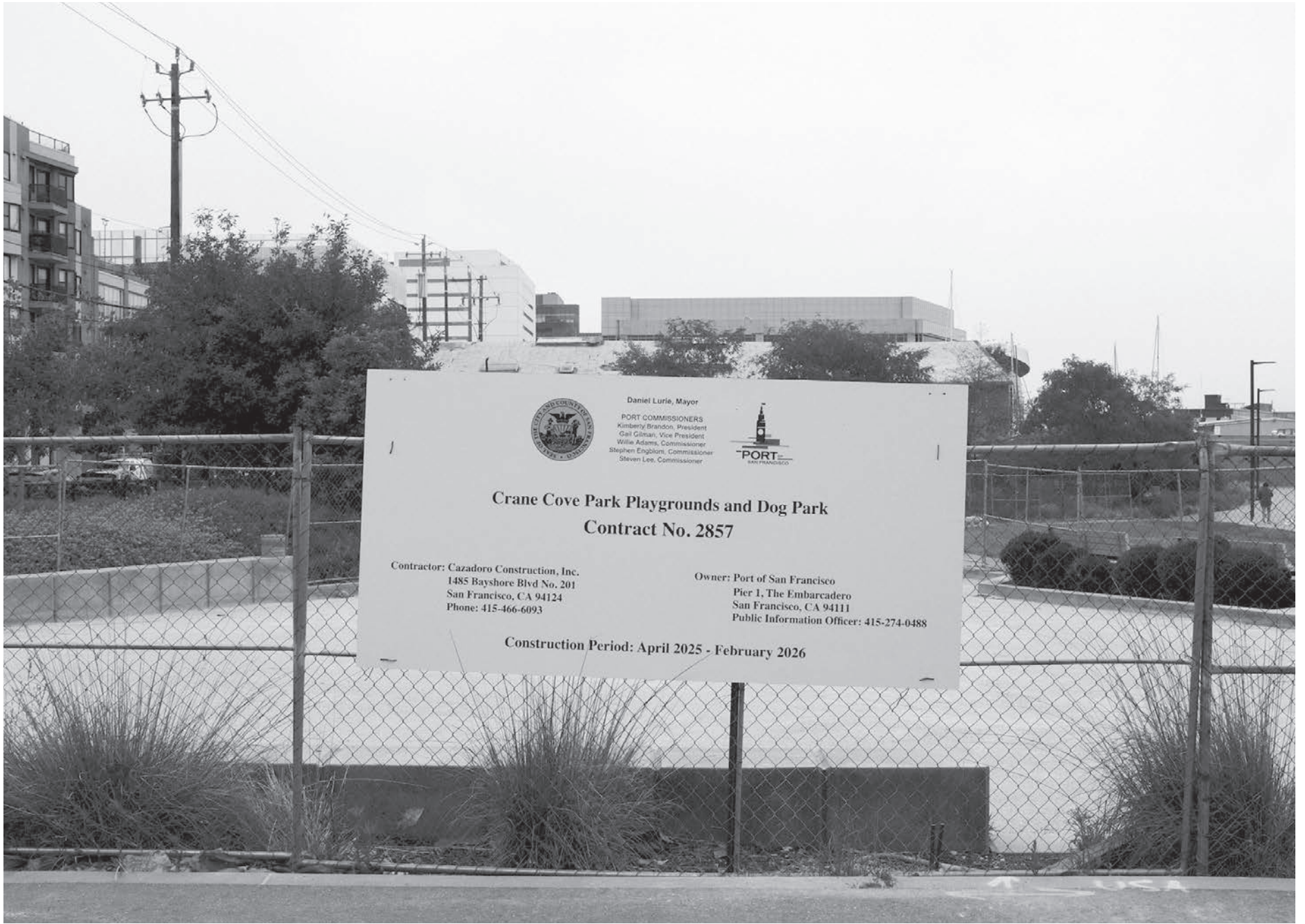
A new playground is being constructed in front of the Dogpatch YMCA at Crane Cove, with an estimated completion date of February 2026.
