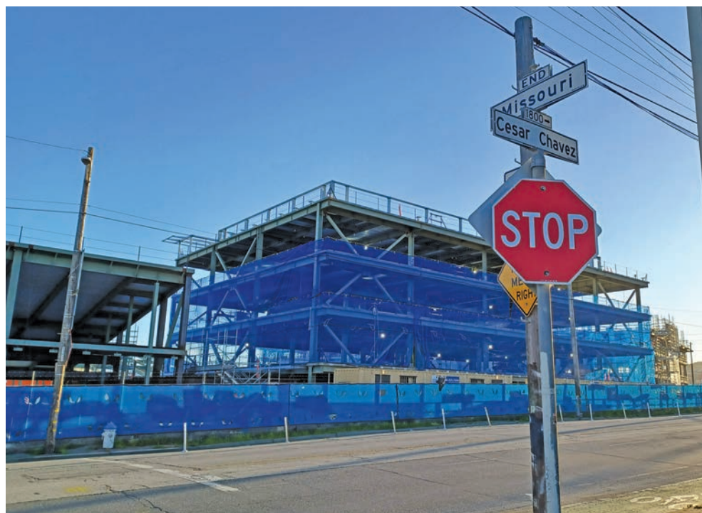
San Francisco Public Utilities Commission's Water Divisions Operations Center's new 371,000-square foot facility is under construction at 2000 Marin Street. PHOTO: Jessica Zimmer
